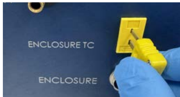
Figure 6: Connection of Type-K thermocouple to chiller unit
