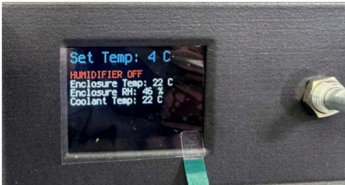
Figure 12: Front panel user display for chilling unit directly after powering on
